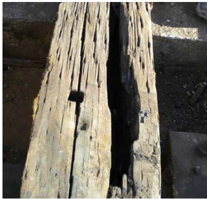
Top-Left: Original rail ties from the 1970's can be found throughout the core system. These must be replaced. Bottom Left: 90 miles of original rail is worn down from 40 years of use. Right: BART crews work to repair worn tracks in the Transbay Tube.
