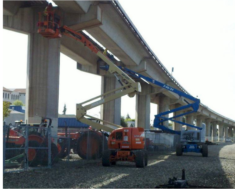
Left: Equipment in 42 of BART's 56 electrical substations require rehabilitation. Right: Traction power cables throughout the system require upgrades.
