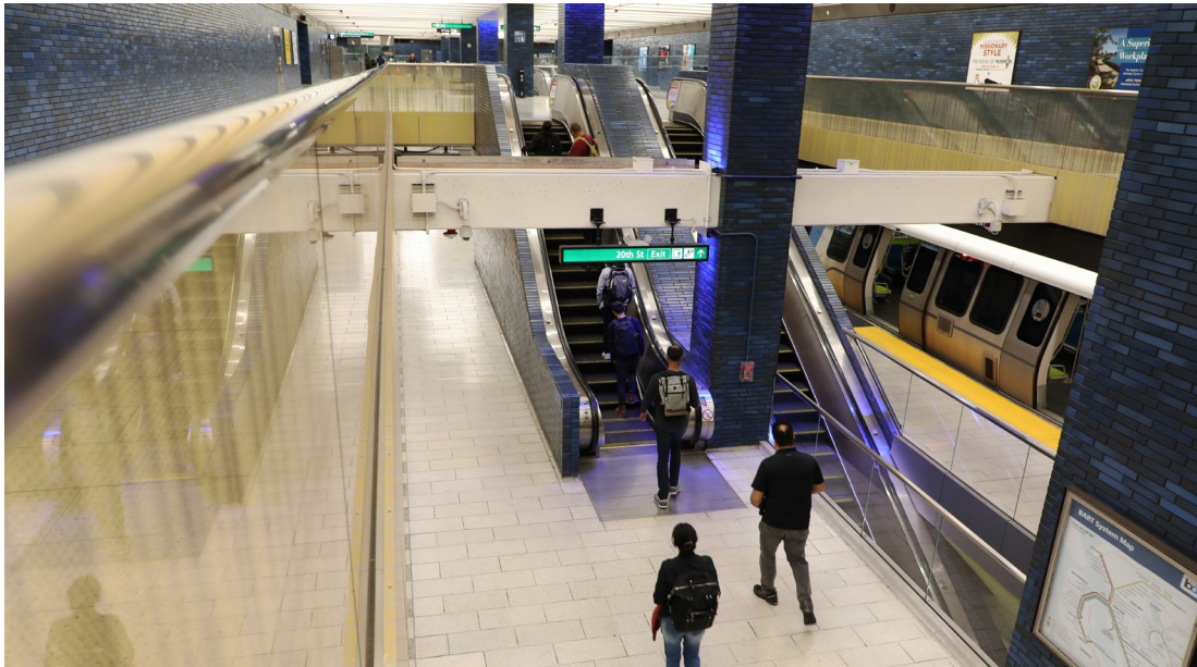
New energy-efficient LED lighting helped brighten the concourse and platform areas of 19th Street/Oakland Station.
