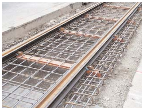
An example of the track construction is shown in the image above.
