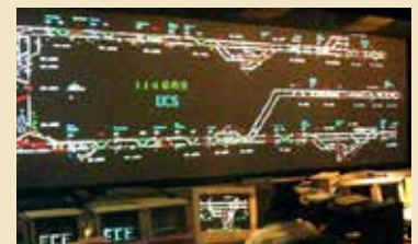
BART's existing Operations Control Center
