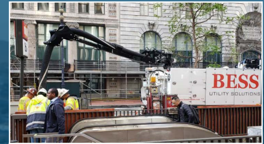
MARKET STREET ESCALATORS (15LK-120)
