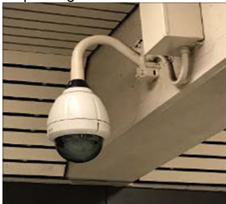
Sample Image of Semi-Visible CCTV camera
