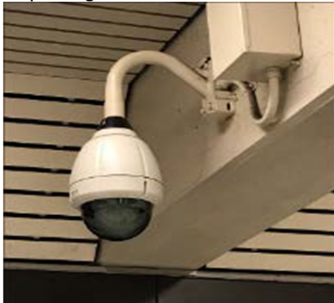
Sample Image of Semi-Visible CCTV Camera
