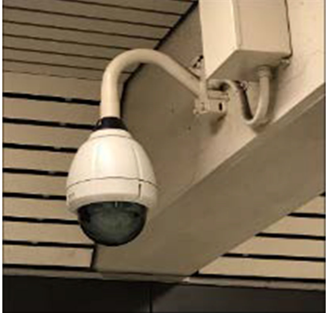
Sample Image of Semi-Visible CCTV Camera
