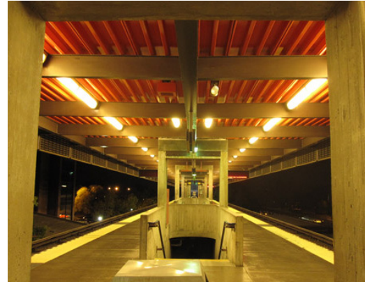
EXISTING CANOPY LIGHTING GLARE
