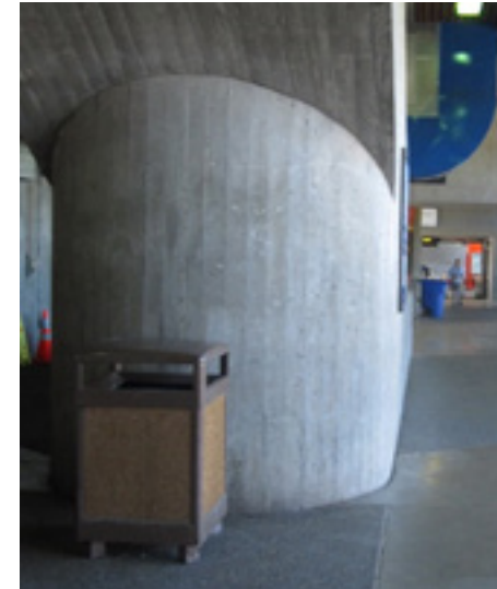
Non-structural, Over-sized Concrete Escalator Cladding
