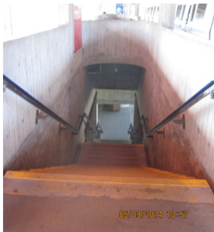
No top of stair tactile warning
