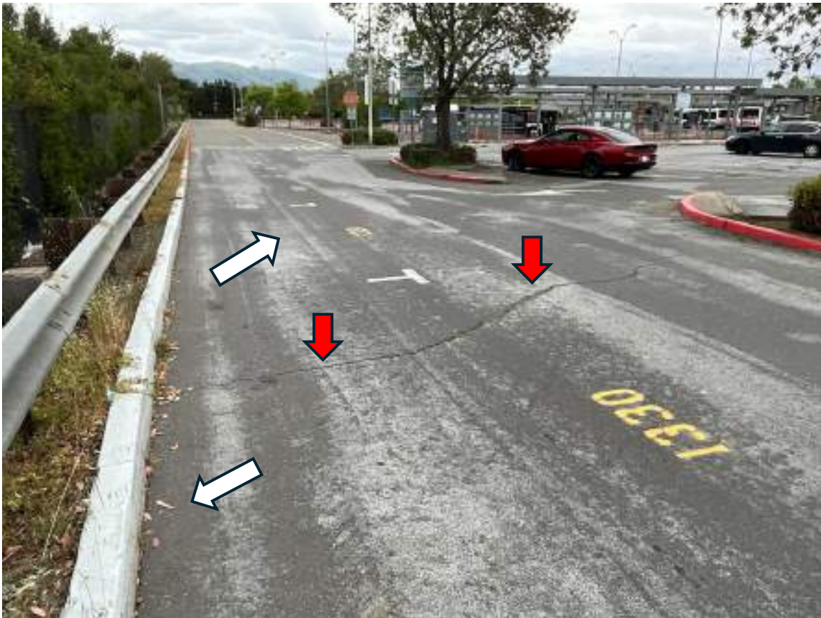
Photo 1: View to south along eastern access road within Parking Lot H. Note offset curb (white arrows) and cracking in pavement (red arrows).
