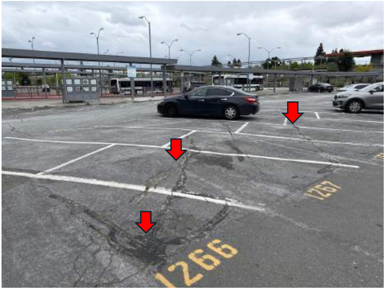
Photo 2: View to southwest of pavement cracking (red arrows) within Parking Lot H coincident with mapped creeping trace of the Hayward fault (Lienkaemper, 1992).
