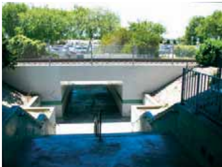
The pedestrian underpass lacks visibility and has hiding places.
