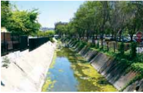
The Estudillo Canal that separates Bayfair Center from the Bay Fair BART station.
