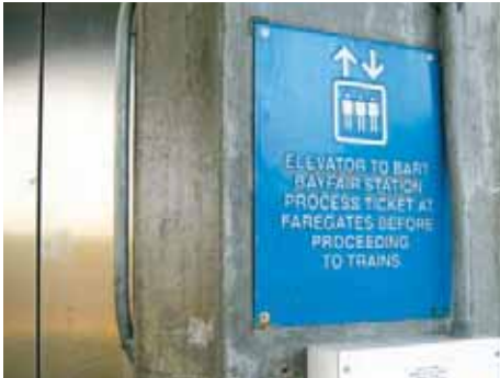
A new honor gate at the elevator entrance would facilitate easier elevator access for patrons with mobility needs.
