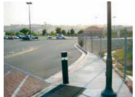
The sidewalk along Bayfair Drive is incomplete.
