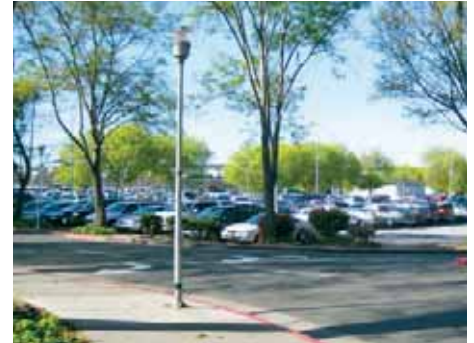
Broken lamps on existing light standards.
