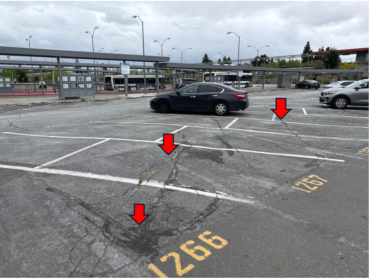
Photo 2: View to southwest of pavement cracking (red arrows) within Parking Lot H coincident with mapped creeping trace of the Hayward fault (Lienkaemper, 1992).
