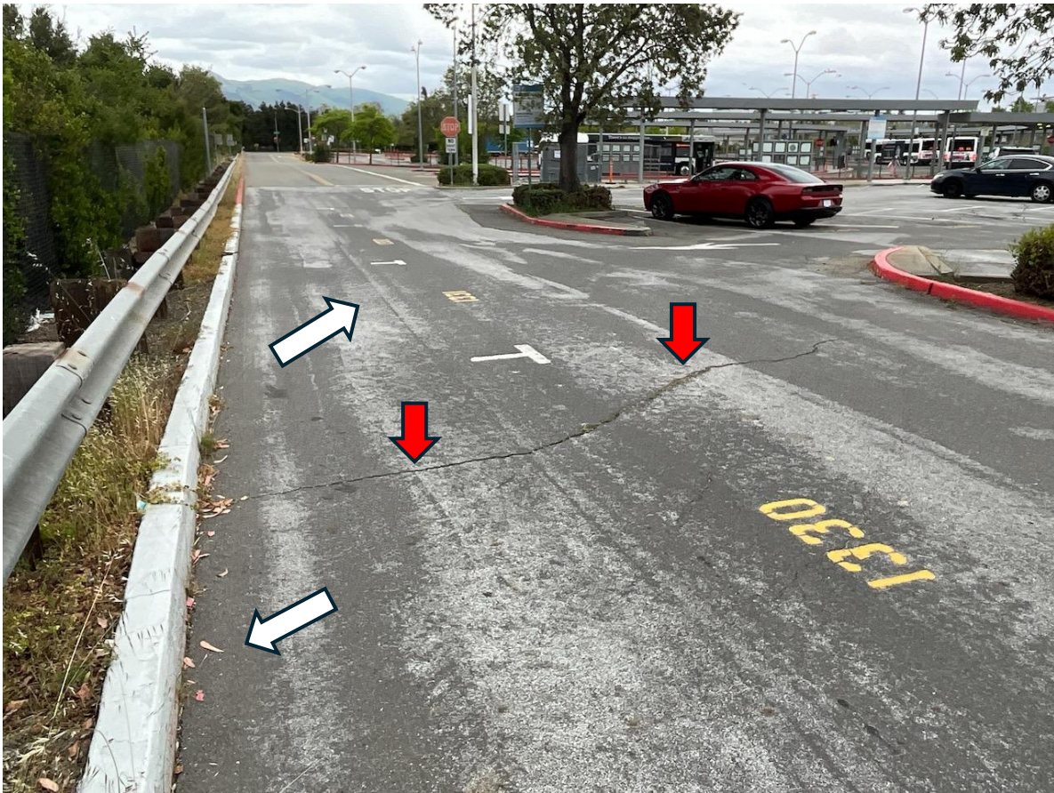
Photo 1: View to south along eastern access road within Parking Lot H. Note offset curb (white arrows) and cracking in pavement (red arrows).
