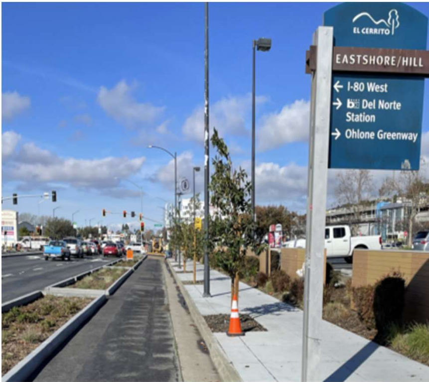
During Construction near the El Cerrito del Norte BART Station for Improved Bikeways
