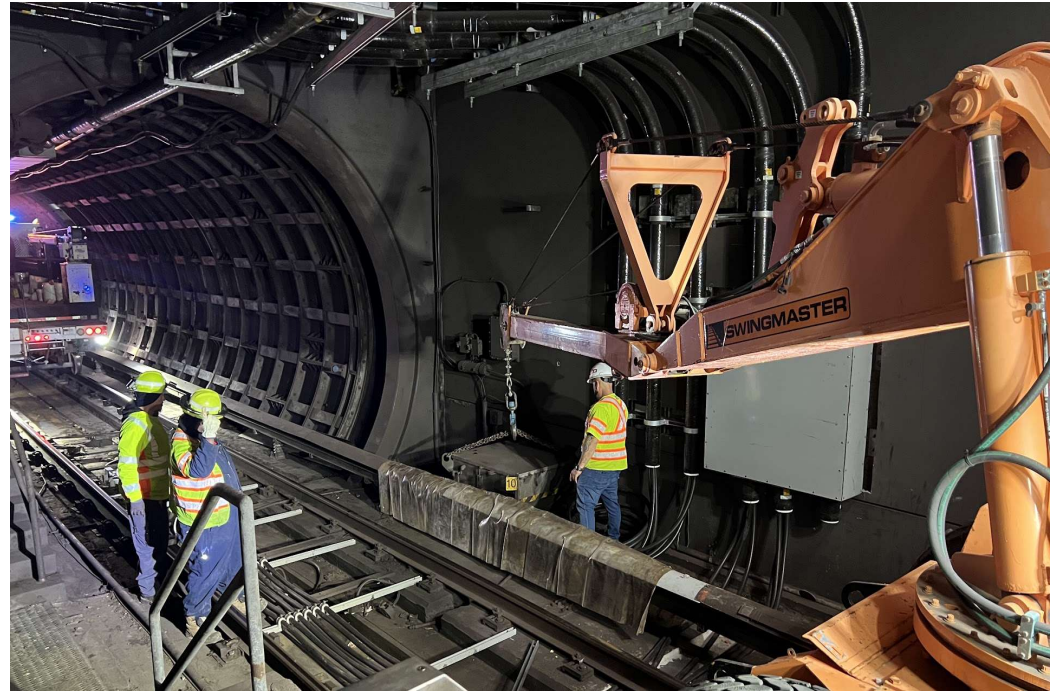
Construction Crew Connecting Traction Power Cables with 3 rd Rail at Montgomery Station
