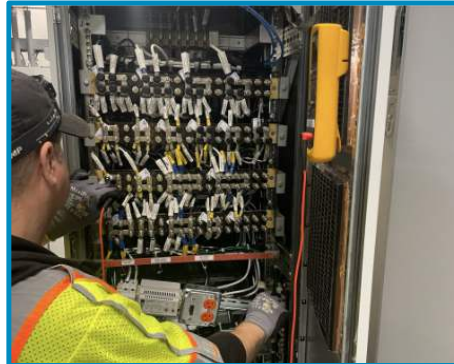
Colma Train Control Room Testing
