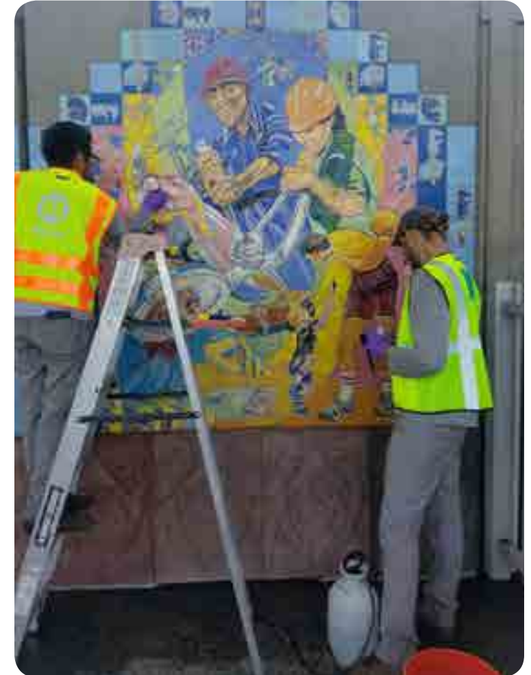
LA Metro and the RLA Conservation staff working together to repair artworks at the Slauson Station. Photo: RLA Conservation
