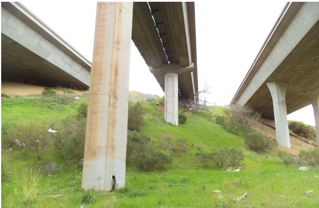
Note: Project site is the middle structure and the slope below, as viewed from Kinne Blvd., looking west. Figure 10. View of Concord Project Site C3015W
